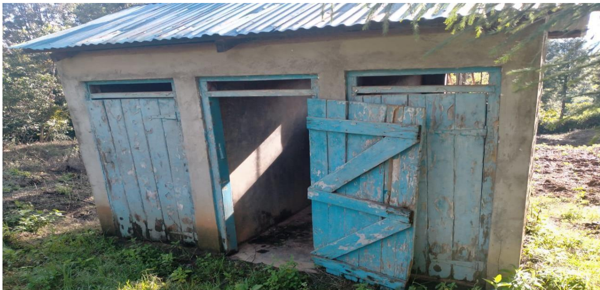
Figure 4: Teachers' latrines (own photo)
