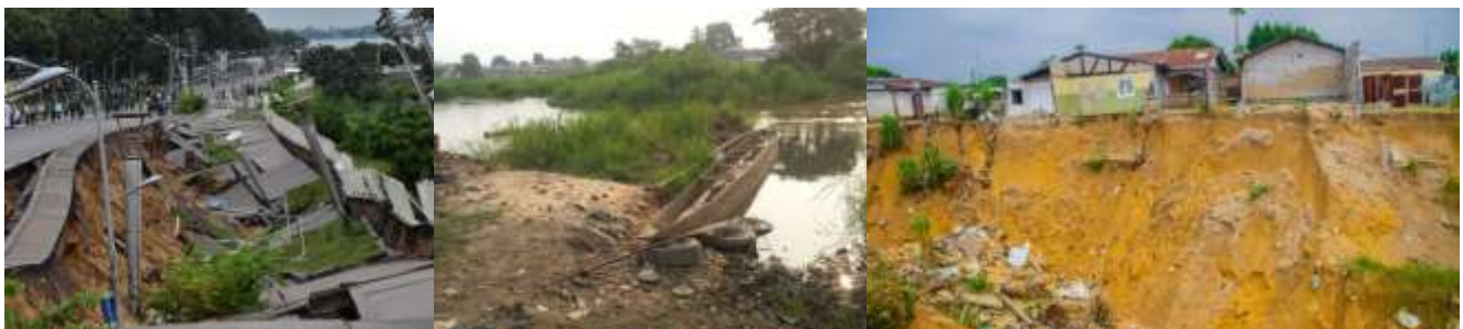
Photo 1: Erosion processes observed on the banks of the Tsiémé River
