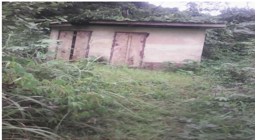
Figure 2. An unkempt latrine facility in a village primary school of Mundemba subdivision
