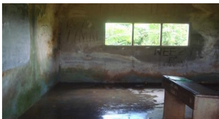
Figure 2. Deserted classroom in need of repairs in Mundemba subdivision
