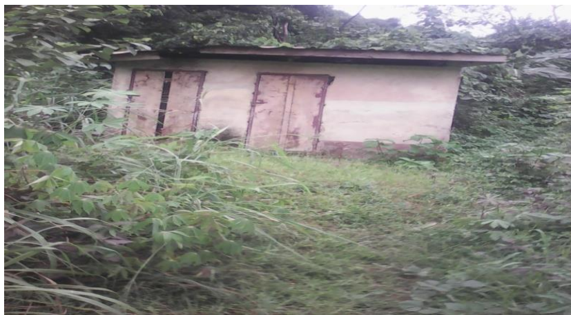
Figure 2. An unkempt latrine facility in a village primary school of Mundemba subdivision
