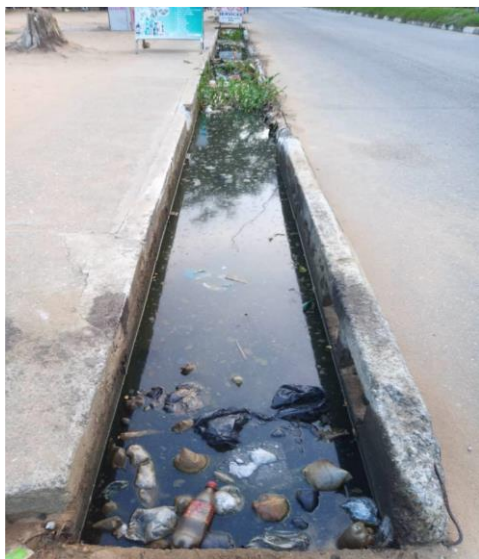
Plate I: Poor drainage condition at Abak Road
