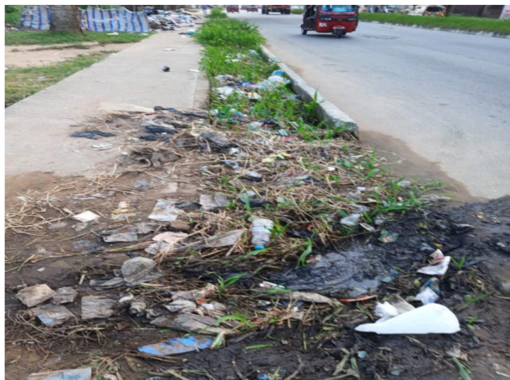
Plate II: Blocked Drainage at Nwaniba
