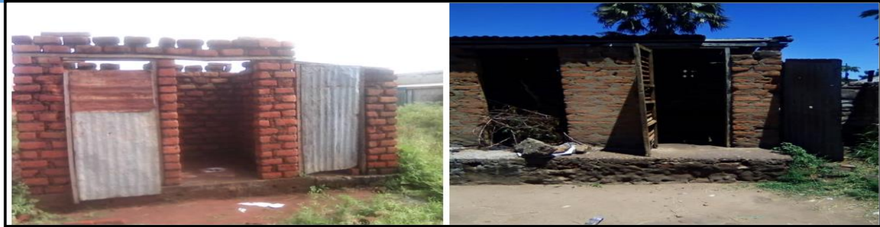
Figure 4: latrines without locks, lights, doors and roof. Photo credit: Okot
